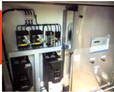
The lift station is the first in the state to be controlled by a Flygt SCADA system.
