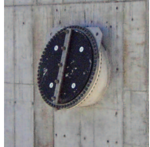
This 84" Waterflex was installed in the inlet tower of an 1100 acre reservoir.
